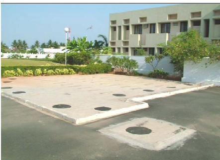
Baffled Reactor of a large DEWATS plant next to a hospital's patient accommodation.
